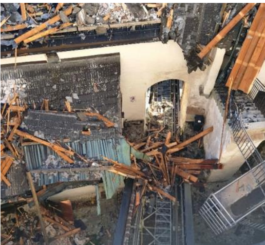
Figure 69 Missing ceiling of the mayor's tower
